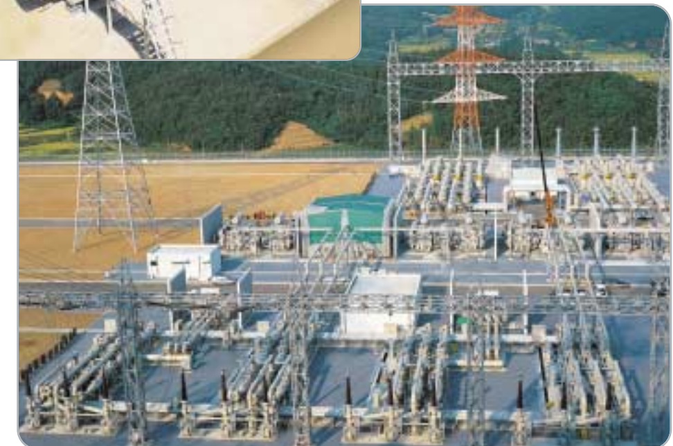
362kV & 800kV GIS under Commercial Operation
