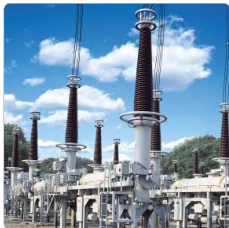
362kV GIS under Commercial Operation
