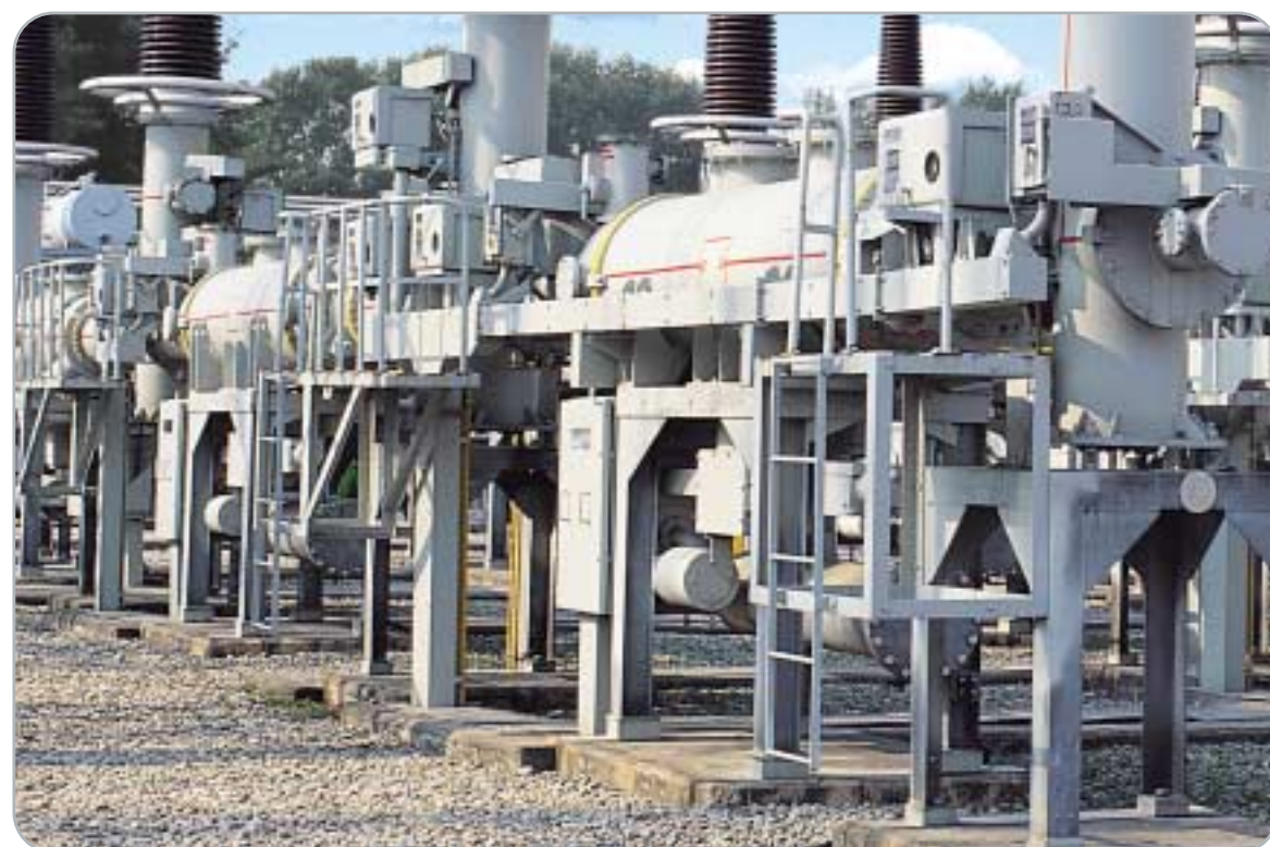
Interlock Systems Installed between Each Equipment
