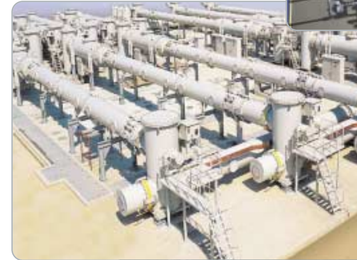
800kV GIS under Commercial Operation
